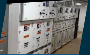
UL 508A & UL 698A Panel Fabrication
