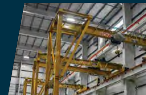
High-Capacity Shops with Bridge Cranes
