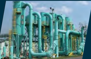
Pneumatic Systems & Process Piping
