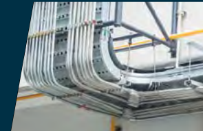
Complete Electrical Installation
